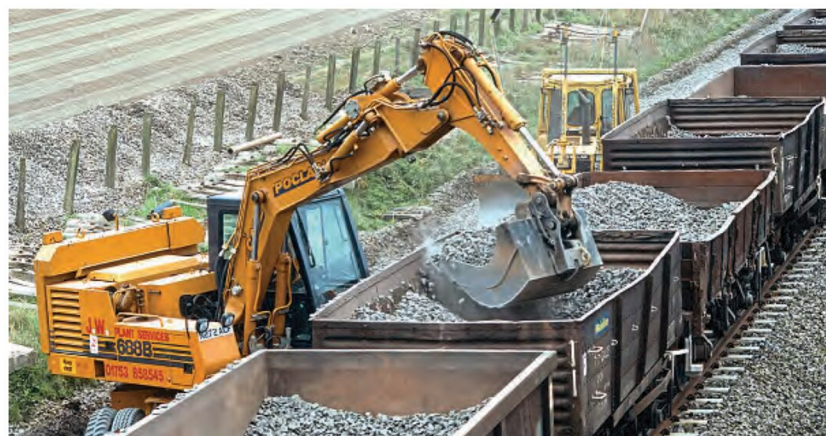
The battered condition of many older vacuum braked ballast and spoil wagons can be explained by this picture. The train, which was photographed near Hungerford, consists of quite a mix of wagons including one 'Grampus' with quite bowed and damaged sides. It is a 'Dace' that is being unloaded.
